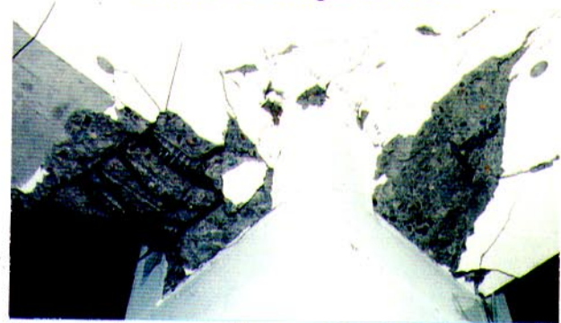
Photo 5. Damaged Girders of 1st RC Frame
