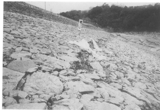
Photo. 3 Shallow sliding at the upstream slope of Kitayama Dam No.1
