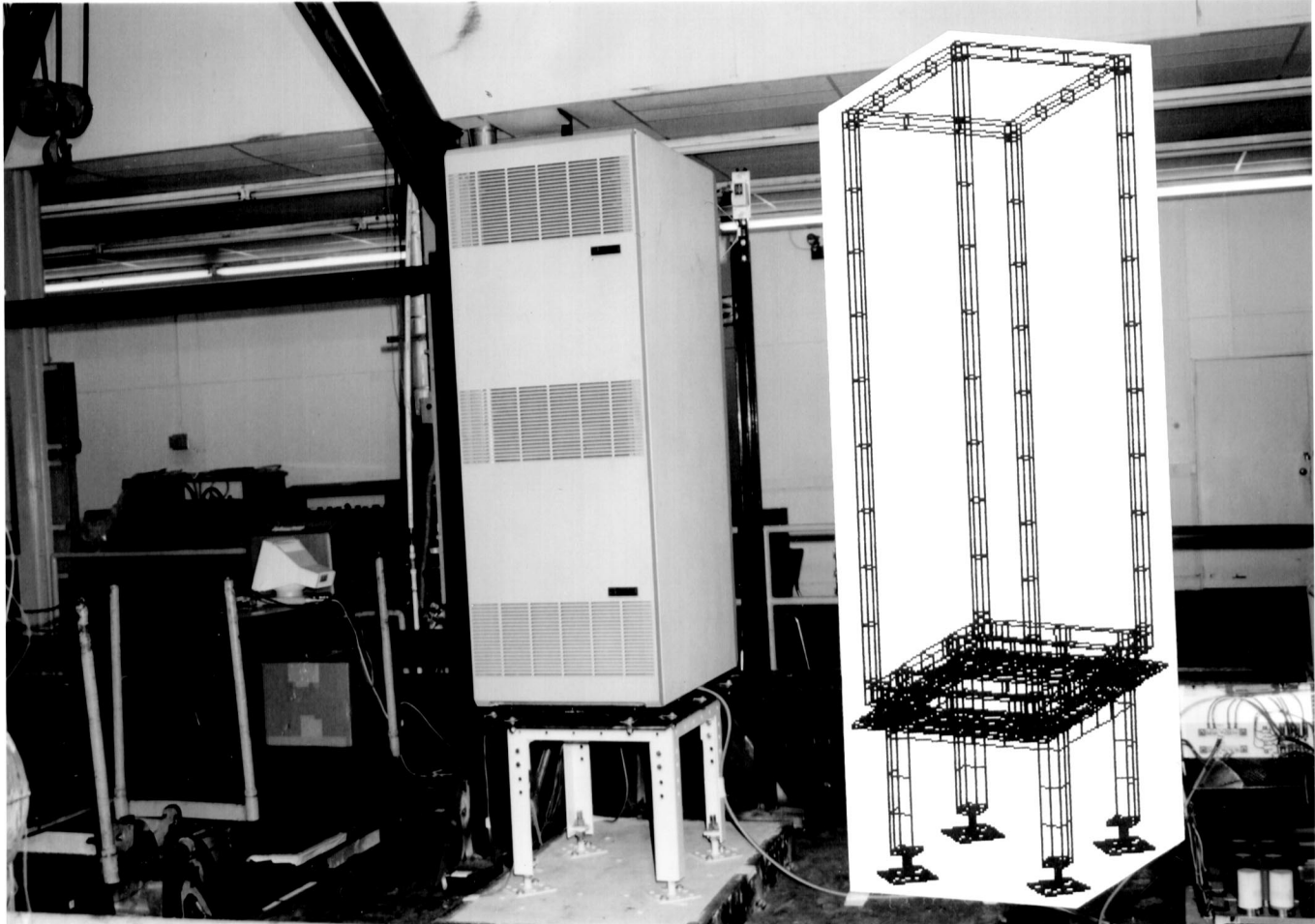
FIG. 3. Pedestal mounted finite element model and telecommunications equipment on seismic simulator.
