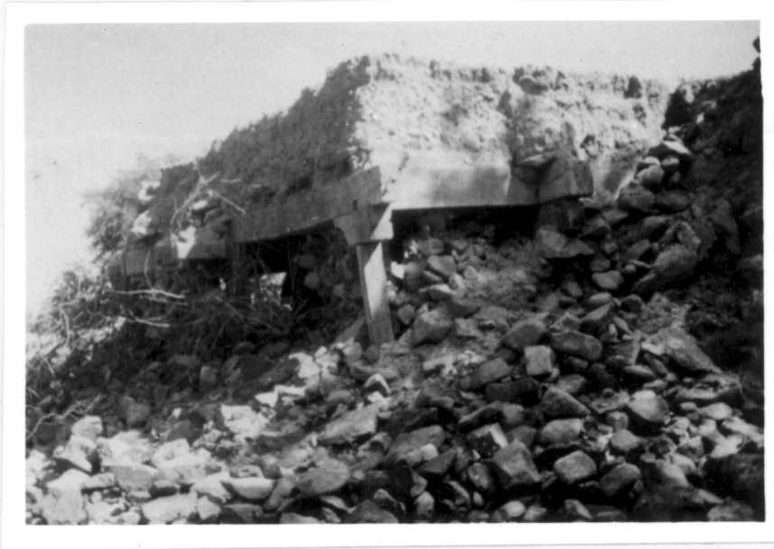
Photograph 1. Timber frame structure.Thick over burden of soil on top. Shattered walls. These were constructed in non-engineered stone masonry with mud mortar.
