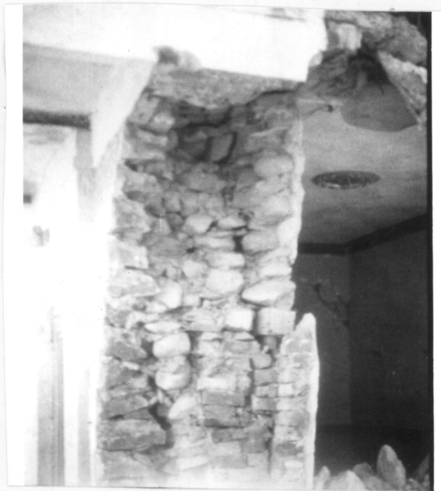
Photograph 2. Typical cross section of wall. Wall constructed in mud mortar. All sorts of stones,brick bats are used. No through stones.
