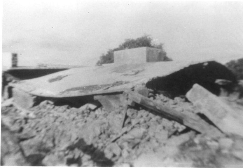
Photograph 3. Collapse of slab due to failure of walling system.
