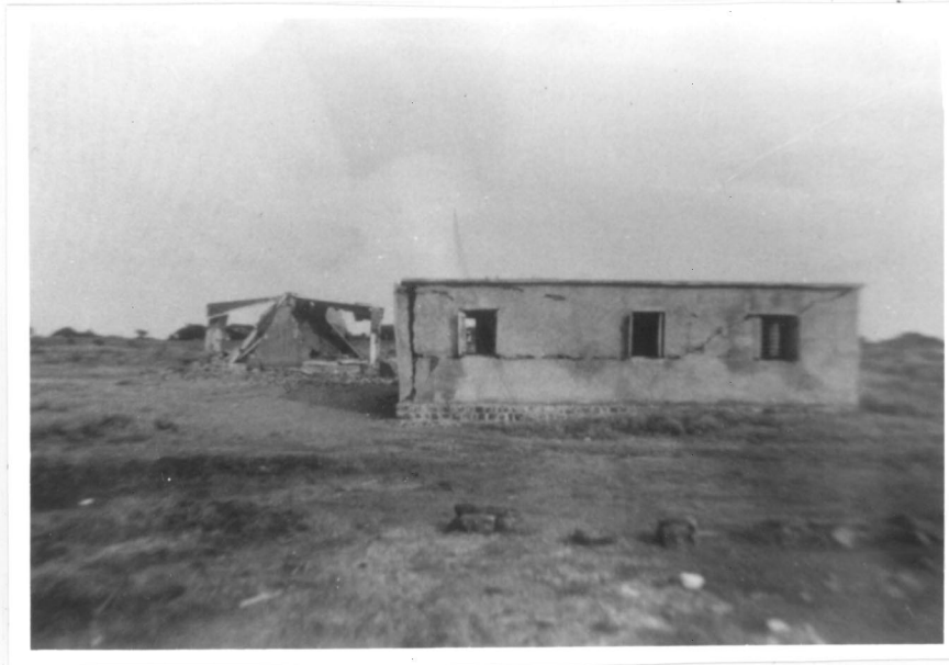
Photograph 7. damage to school building due to long walls without columns & horizontal bands
