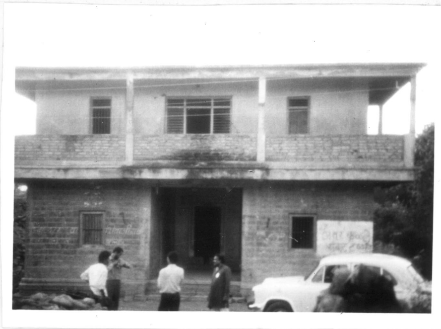
Photograph 6. Two storeyed intact building at Sastur constructed with good quality stone masonry, though no bands were provided. (At 7 km from epicentre)
