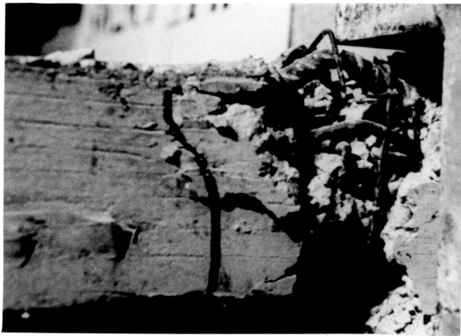
Fig. 11. Wall SW23C1 - rupture of stirrups at ultimate state
