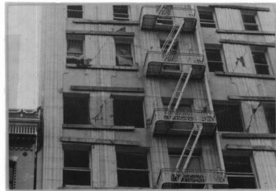
Fig. 2. Damage of Contact Region and Masonry Pier on South Face of 10-Story Building.
