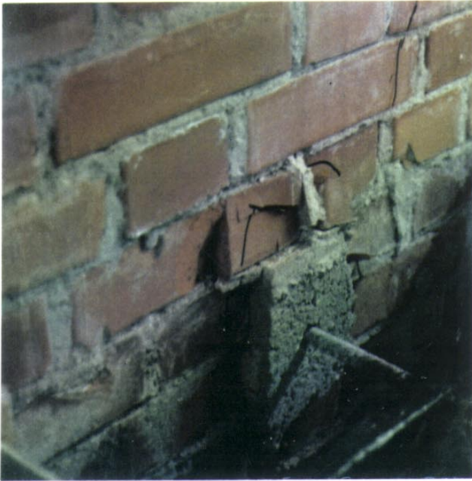
Fig. 8 Picture of anchorage type A at collapse.
