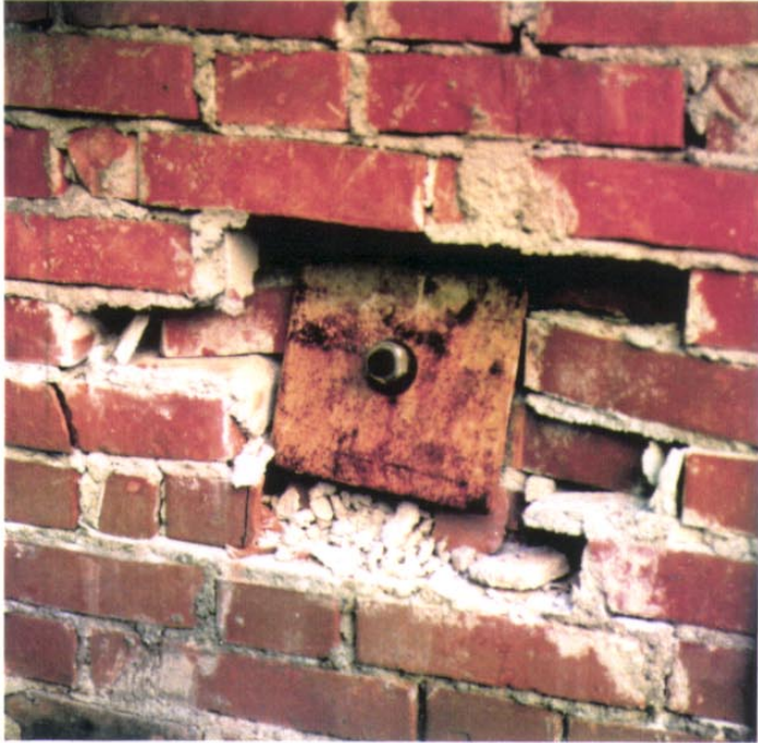
Fig. 11 Picture of anchorage type C at collapse.
