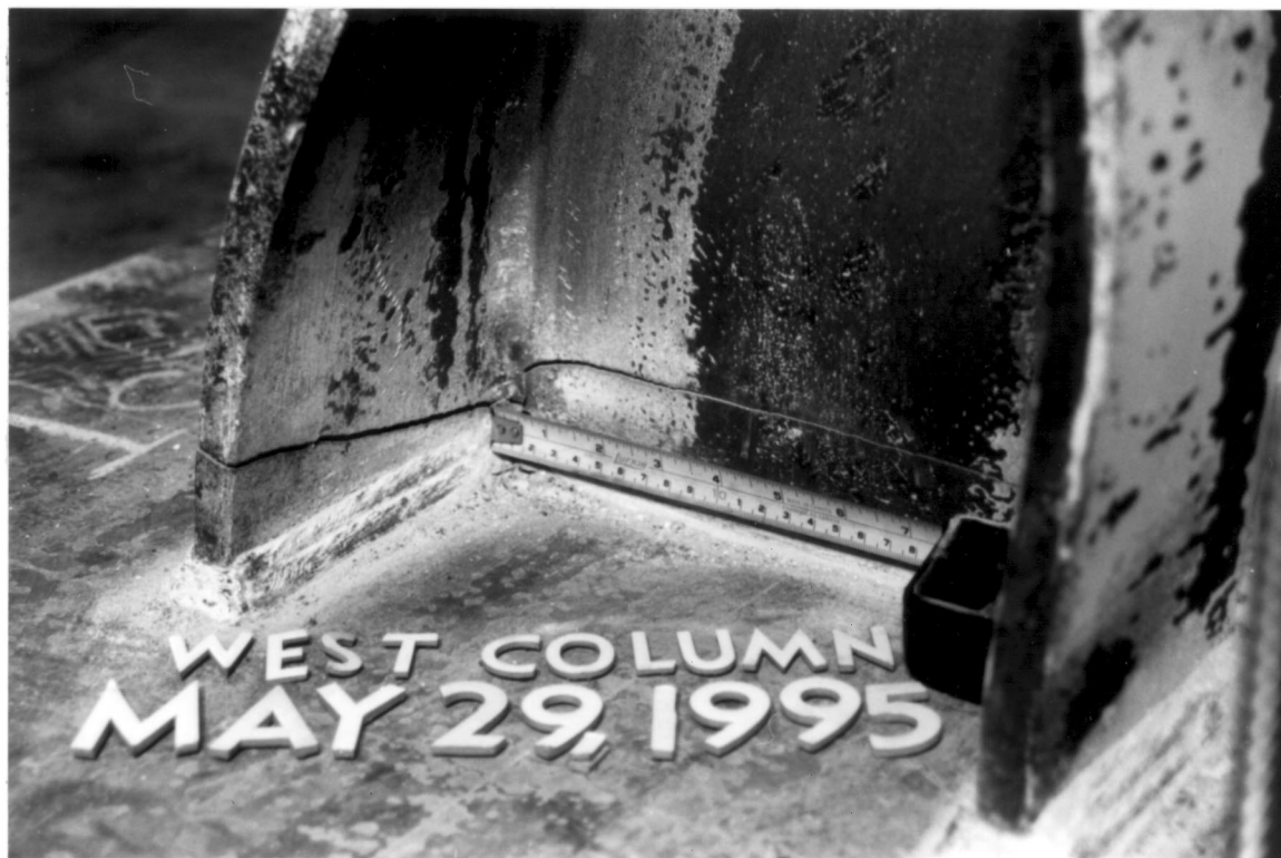
Fig. 7 Fractured West Column
