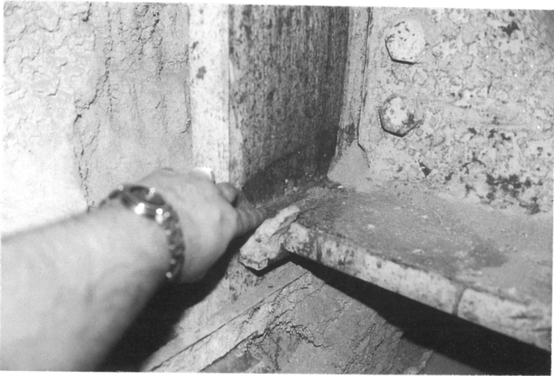
Figure 3. Beam-column connection damage.
