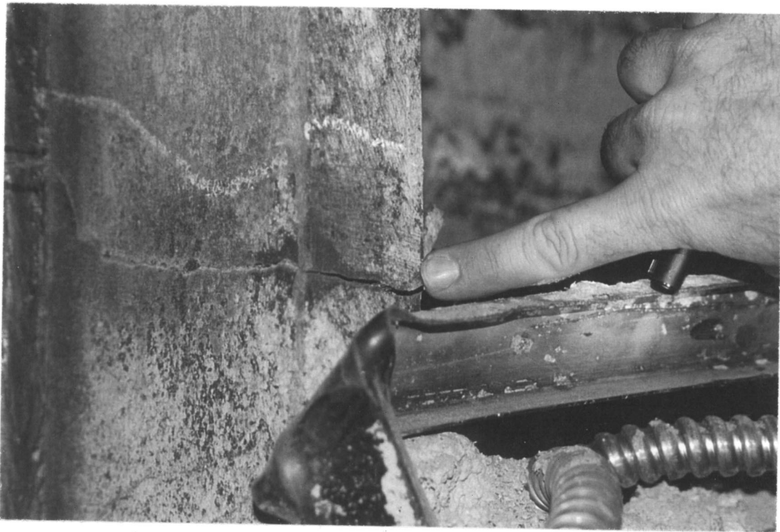
Figure 4. Beam-column connection damage.
