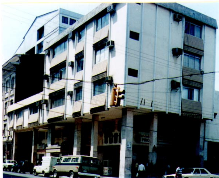
Fig. 3. Difference in stiffness between first and upper floors in a building at Guayaquil city. After Ruffilli.
