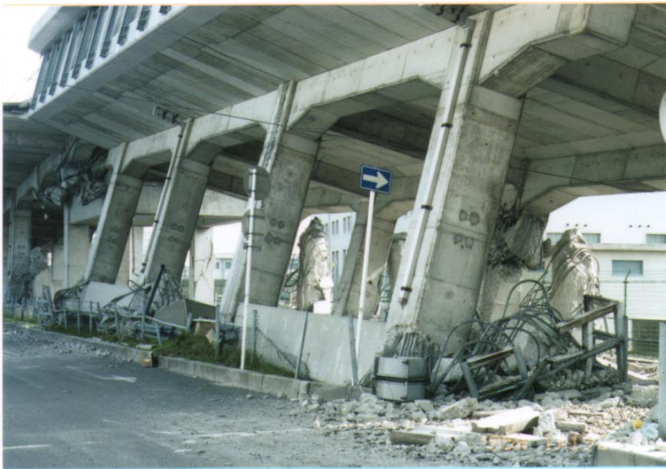
Photo 1 Damage to RC Viaducts Due to 1995 Hyogo-ken Nanbu Earthquake
