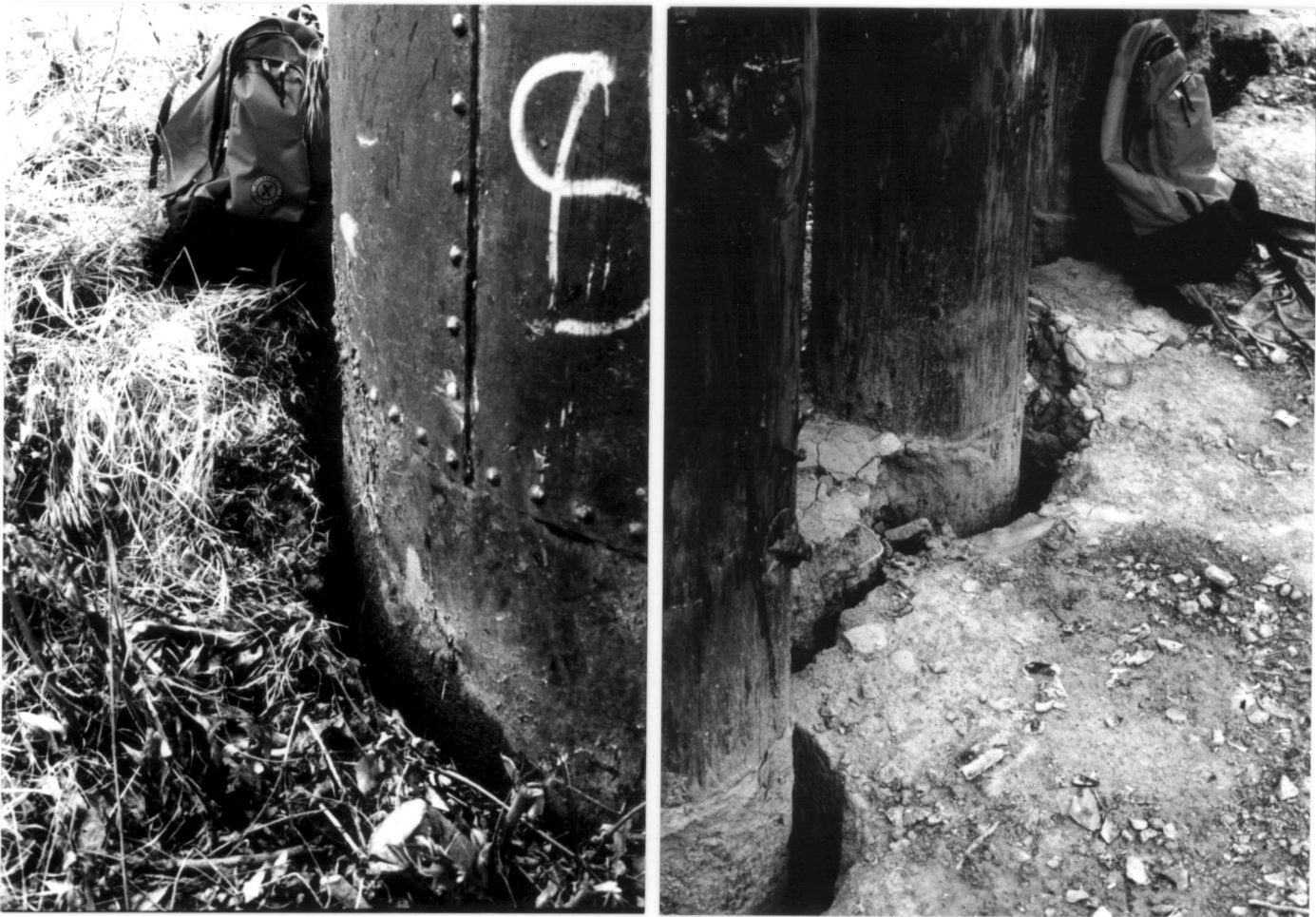
Fig. 1 Gapping adjacent to bridge piles near Watsonville after the Loma Prieta earthquake. Left a large diameter pier near the middle of the bridge; right smaller diameter timber piles in the approach span.
