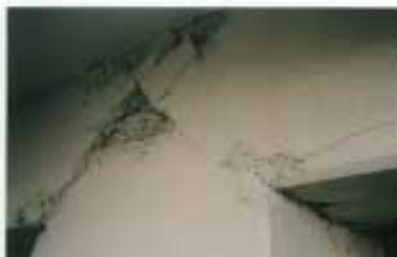
Photo 5 Damage of Beam-to-Column Connection
