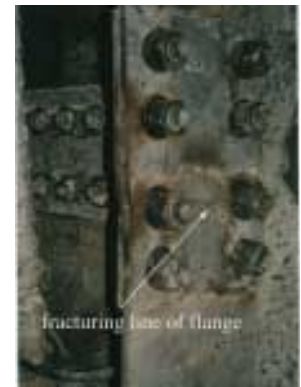
Photo 7 Fracturing of Splice Plate at Column Joint (after chipping concrete)
