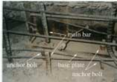
Photo 3 Fracturing of Anchor Bolt at Column Base (after chipping concrete)
