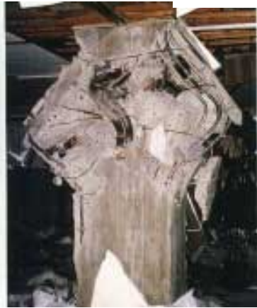
Photo 2 Collapsed Column in Shear
