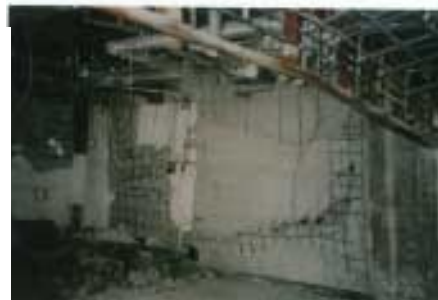
Photo 6 Damage of RC Shear Wall
