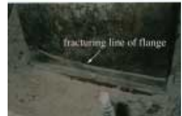
Photo 4 Fracturing of Column Steel Flange Plate (after chipping concrete)
