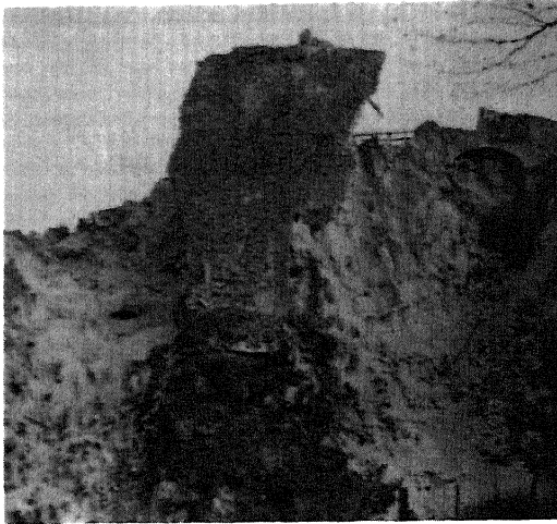
Figure 1. View of the bastion after the collapse
