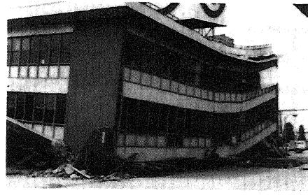
Photo 3 Collapse of soft-first-story type building (Off-Miyagi prefecture earthquake, 1978)
