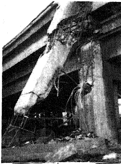
Photo 1 Collapsed Cypress Interstate double-deck bridge in California (Loma Prieta earthquake, 1989)
