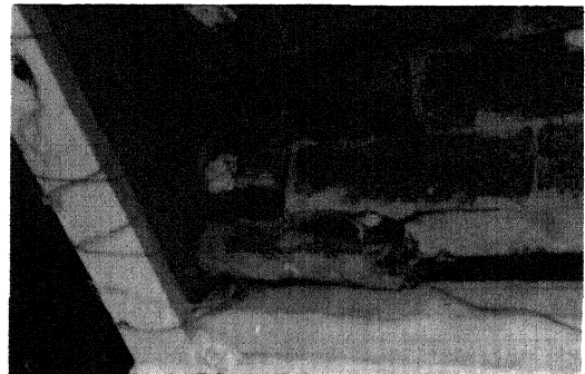
Figure 9b. Detail of damage
