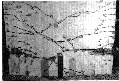
Figure 7. Unit after failure.
