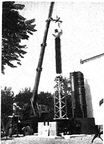
Figure 7. 500 KV Current Transformer erected over the shaking table for testing.
