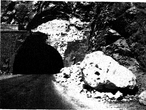
Figure 2. Cracks and partial collapse of the concrete and stone masonry facing in Manjil Tunnel entrance.
