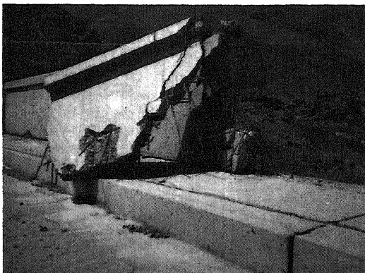
Figure 11. Damage of the parapet walls on the Sefidrud dam's crown.
