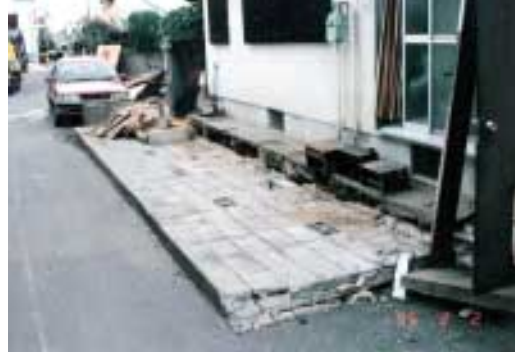
Figure 1: Structural damage to a masonry garden wall by the 1995 Hyogoken-nanbu earthquake
