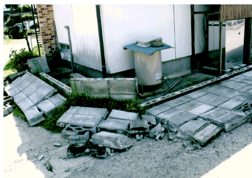
Figure 4: Structural damage to masonry garden walls by the 1997 Kagoshimaken-hokuseibu earthquake
