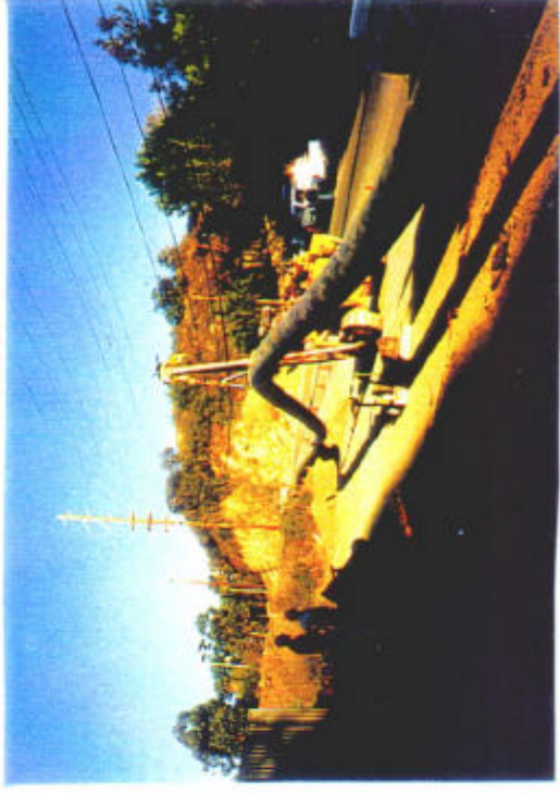
Figure 4-500 mm OD x 50 mm (20-in OD x 2-in) HDPE pipe laid on roadway prior to insertion into 300 mm (12-in) cast iron pipe. (L. Lund)
