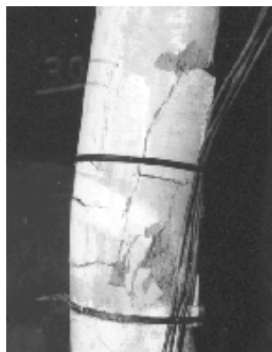
(b) Damage of middle part of pile
