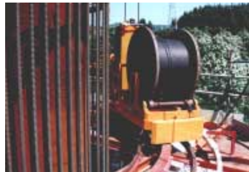
Figure 19: Automated spiral strand feeder
