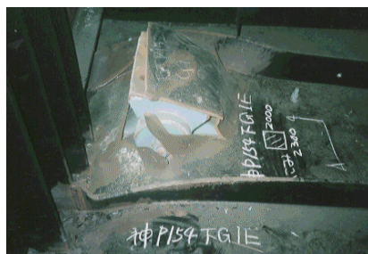
(a) Bearing's penetration into lower flange
