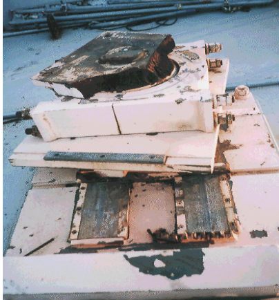
(c) Broken bearing
