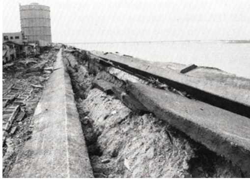
Photograph 1: Damaged to the Torishima Dike [Matsuo, 1996]
