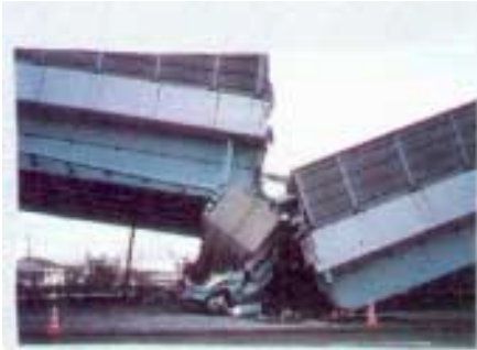
Photo 1 Collapsed bridge pier
