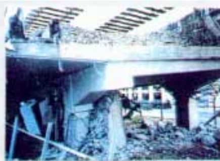
Photo 2 Collapsed viaduct pier
