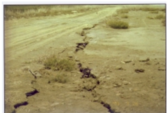
Fig. 5 Cracks damage on country road
