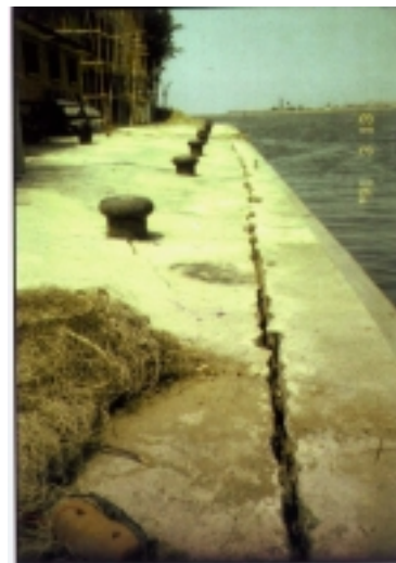
Fig. 4 Damage in Masago harbour
