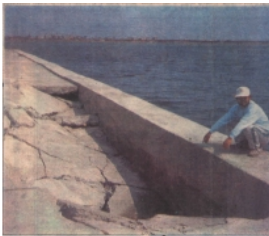
Fig. 4 Damage in Masago harbour
