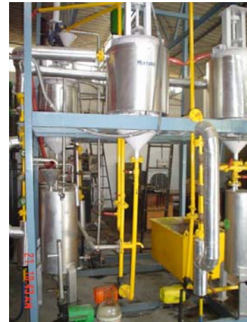
The Engine Research Lab, Biodiesel Pilot Plant (25 Litre/ batch)
