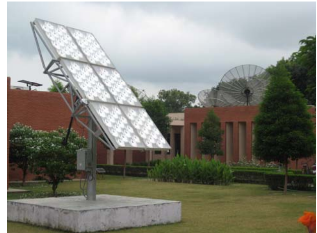
A 1.2 kWp solar concentrator PV system Installed by Moser Baer on IIT campus.
