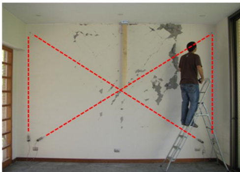
Figure 3.14 Instrumentation of damaged wall in Building B.
