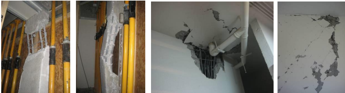
Figure 2.2 a-d(left to right): Structural damage in building 2. From left to right: (a&b) column damage on the ground level floor, (c) wall damage at the underground parking levels, (d) Shear wall damage at ground level
