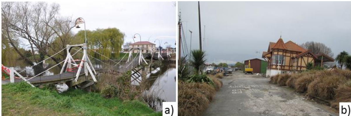
Figure 6. a) Damage to Mandeville footbridge; b) Back-rotation of the Kaiapoi Visitors Centre
