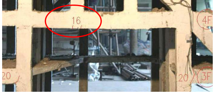
Figure 5.3 Cracks on transfer beam
