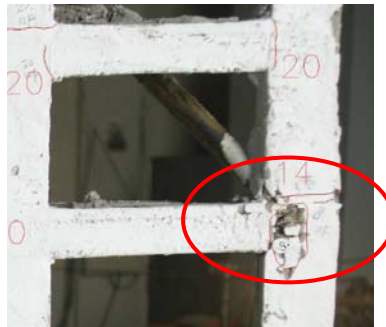
Figure 5.4 Damage of column-brace joint at 11th story
