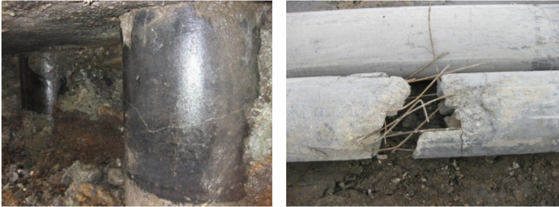
Photo 4. Pile damage of west school building (D14 in Fig. 3) Flexural crack at pile head (left), Partial deficiency of pile at a depth of about 4m (right)
