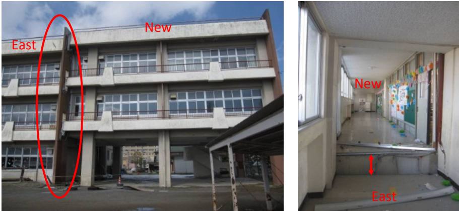
Photo 3. Settlement of east school building (left) and level difference between east and new school building (right)
