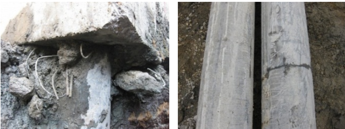
Photo 5. Pile damage of east school building (A9 in Fig. 3) Compression failure at pile head (left), Flexural crack at a depth of about 15m from pile tip (right)
