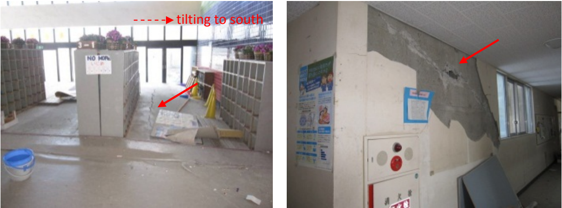
Photo 2. Crack of entrance floor (left) and shear failure of RC non-structural wall in east school building (right)
