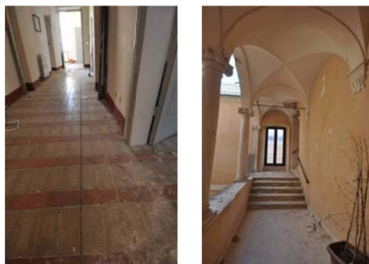
Figure 7. Cracks on the flooring of the first floor and collapse of the "belvedere" of staircase
