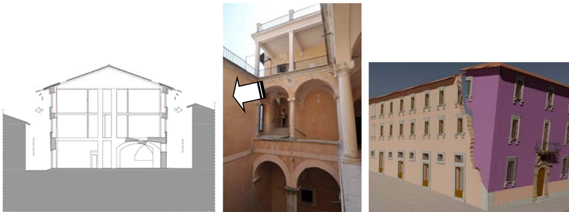
Figure 5. Collapse mechanisms of the lateral façades and of the façade overlooking San Flaviano Sq.
