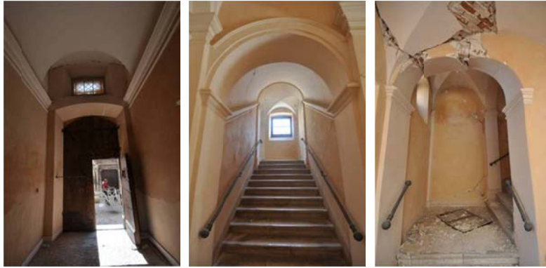
Figure 4. Cracks of the vault on the entry to the courtyard and damage of the vault of the staircase on Sardi St.
