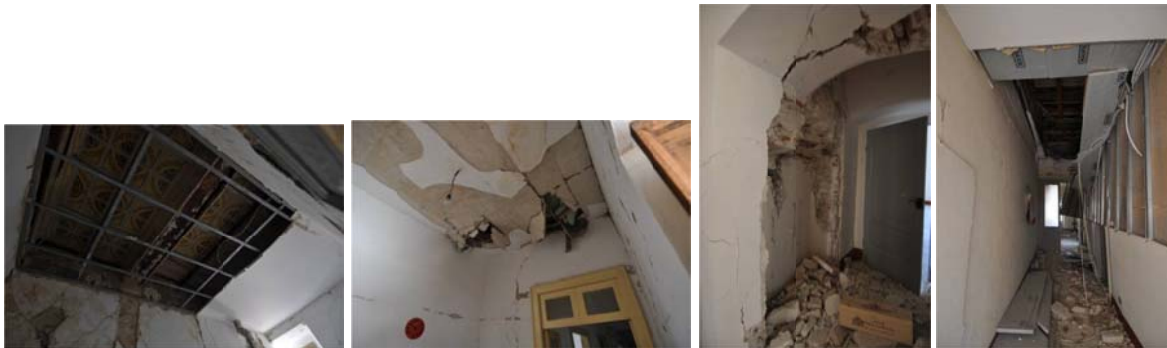
Figure 6. Failure of nonstructural elements: false ceilings and partitions
