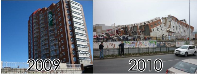
Figure 1.1 Picture of Alto Rio building before and after the Chile earthquake, Feb 2010 (Concepción under Construction, 2010 left; El Periodista, 2010 right)
