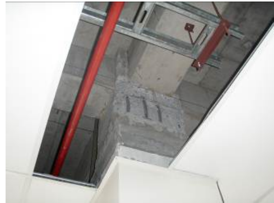
(b) Damage class IV
