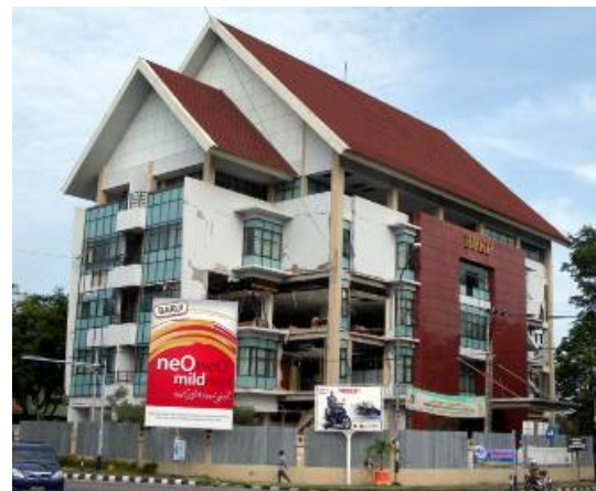
(b) After earthquake damage
