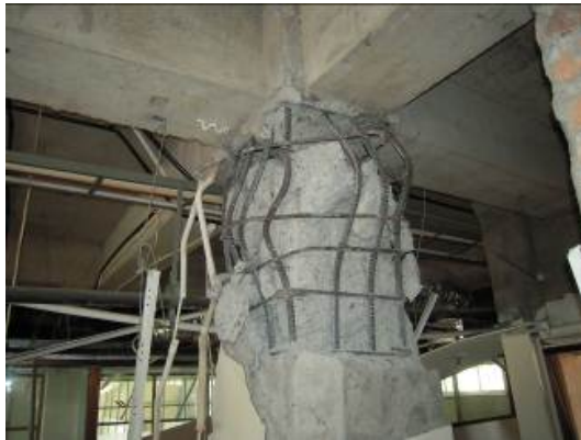
(a) Damage class V
