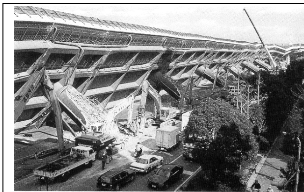
Figure 1. Kobe, Japan, M=7.2, 1995, Total Collapse of Hanshin Line
