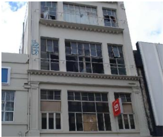
Figure 3. Moderately damages building at Christchurch.
