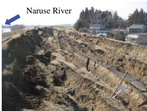
Photo 1. Liquefaction damage caused by the Great East Japan Earthquake of 2011 (river embankment)
