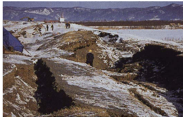
Photo 2. Liquefaction damaged caused by the Kushiro-oki Earthquake of 1993 (river embankment)
