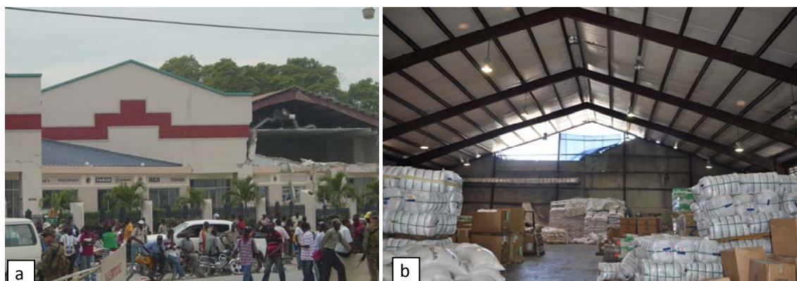
Figure 5. Low-rise masonry infill wall failures of industrial buildings in Haiti a) Gable wall failure of commercial buildings b) Gable wall failure of warehouse building (4b Photo Credit: Steve Baldridge)
