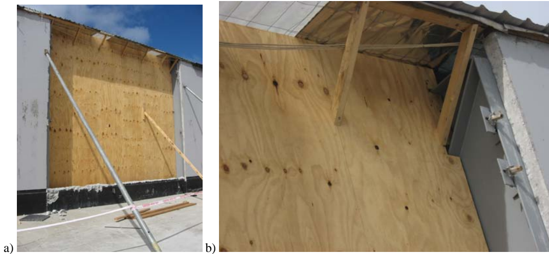
Figure 8. a) Loss of panel and temporary shoring of adjacent panel b) Concrete anchor connection failure.
