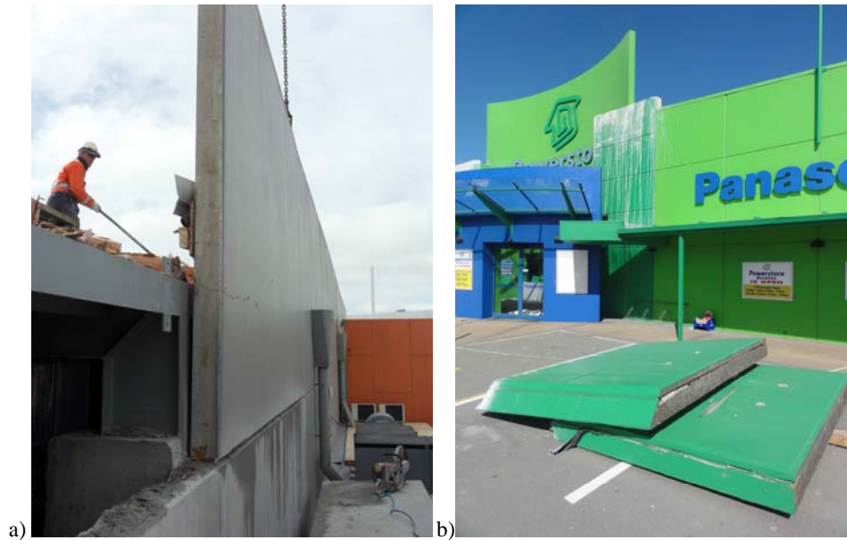
Figure 11. Precast panels with vertical cantilevers greater than 6 ft (1.8m) a) Commercial mall wall panels attached to pre-engineered steel frame b) Commercial tilt-up building.
