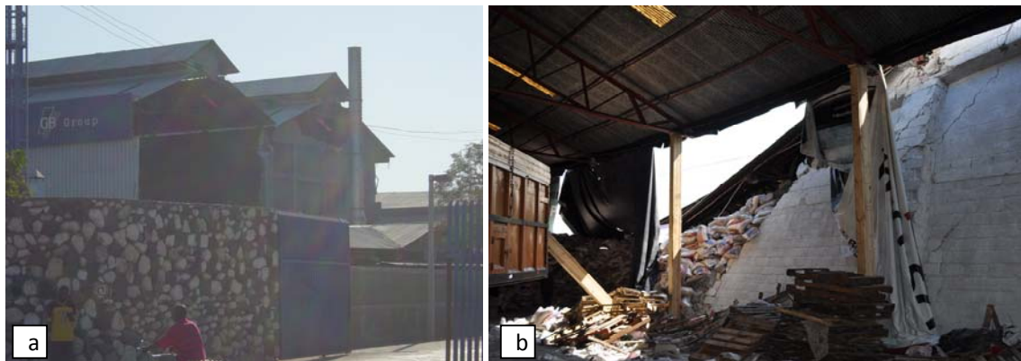
Figure 4. Low-rise masonry infill wall failures of industrial buildings in Haiti a) Endwall failure b) Bearing wall failure and temporary truss supports (3b Photo Credit: Steve Baldrige)
