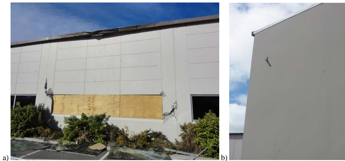
Figure 9. a) Damaged panel due to reduced section b) Cracking of end panel.
