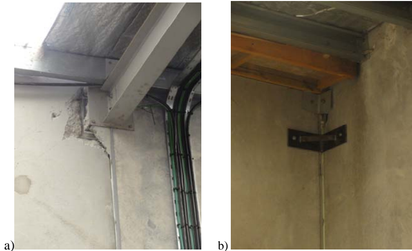
Figure 6. Damaged connections in tilt-up industrial structures in New Zealand a) Beam-to-panel connection damage b) Corner connection damage with post-event repair.
