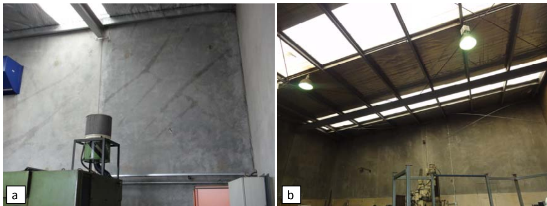
Figure 7. Damaged structural elements in tilt-up industrial structures in New Zealand a) Shear cracking in load-bearing panels b) Fractured tension-only roof diaphragm bracing.
