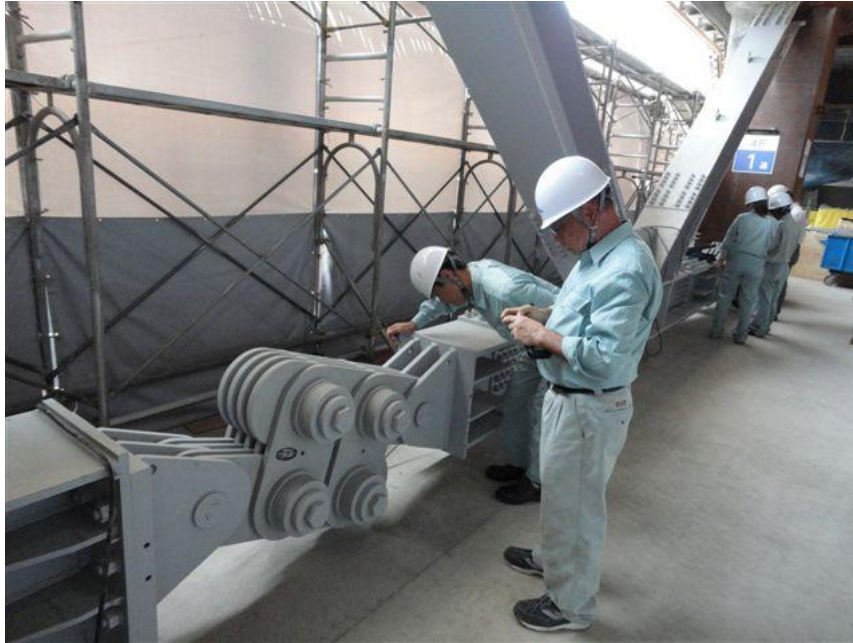
Figure 5. 2250 kN Dampers installed in the building
