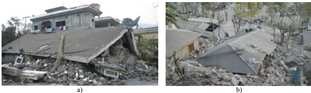
Figure 4.1 Roof collapse due to a loss of the gravity load-bearing capacity of stone walls in the 2005 Kashmir, Pakistan, earthquake: a) reinforced concrete roof, and b) timber and steel roof (photos: M. Tomazevic)
