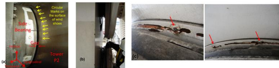
Figure 11. Circular scratch marks on the surface of wind shoe as a result of side bearing movement indicates girder longitudinal movement of about 8cm. (b) Location of head of tower link (P2) bottom head is connected to girder, top head is connected to tower. (c) Scratch marks on the surface of the bottom link head caused by combination of vertical and transverse movement of the girder. The arrows point to locations of three broken bolts caused by the movement.
