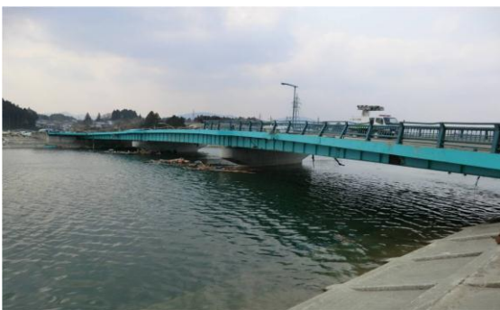
Figure 1.3. Survived the Bridge in Japan (2011)
