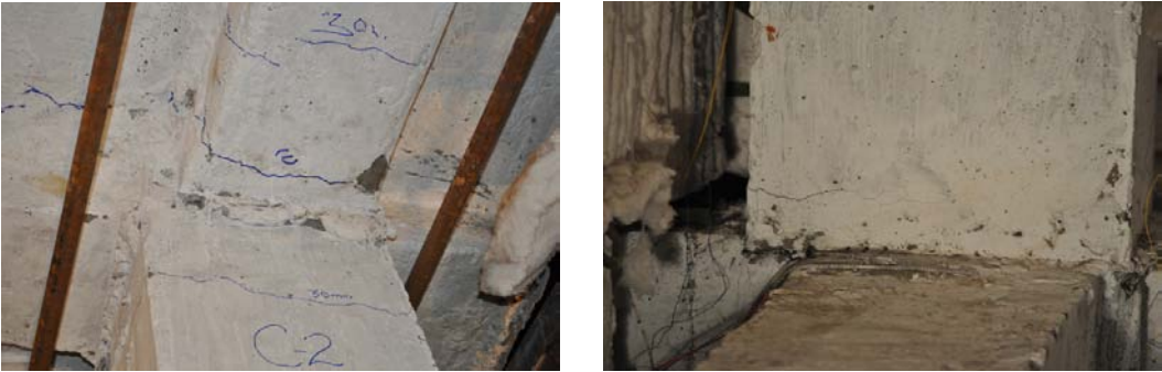
Figure 5 (a). Tension cracks in roof beam B7 (b). Flexural cracking in a column C1
