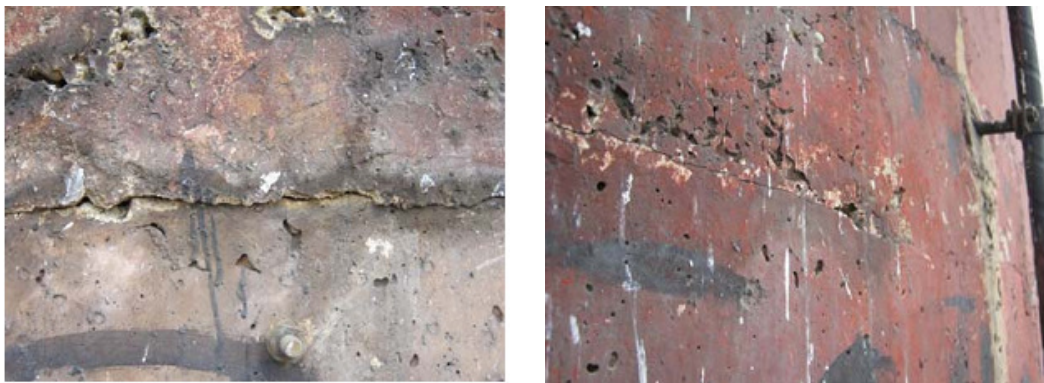
Figure 2. Horizontal cracks at level +142.00
