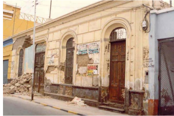
Figure 1.4. Partial collapse of adobe structures. Ica, 1997.
