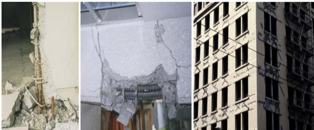
Figure 1. RC buildings failing in shear or bond
