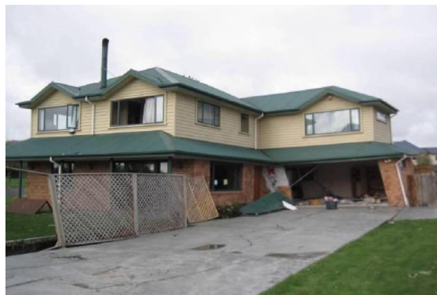
Figure 1. Loss of Integrity at Ground level due to Big Cracks in Concrete Slab
