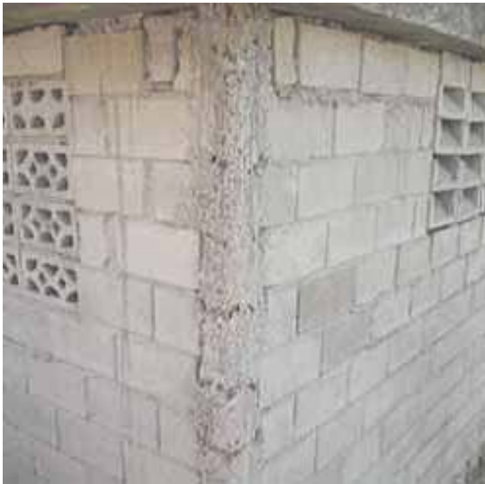
poor concrete consolidation
