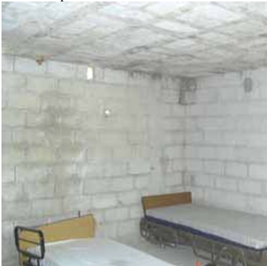
poor workmanship in unreinforced HCB wall
