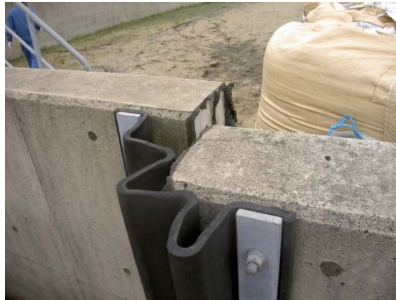
Figure 17. Fracture of wall joint of the dike with rubber sheet protection
