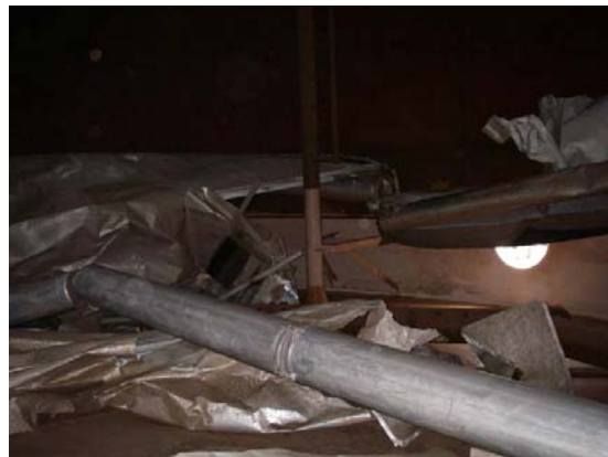
Figure 10. Aluminum inner floating roof of gasoline tank completely broken in Sakata area
