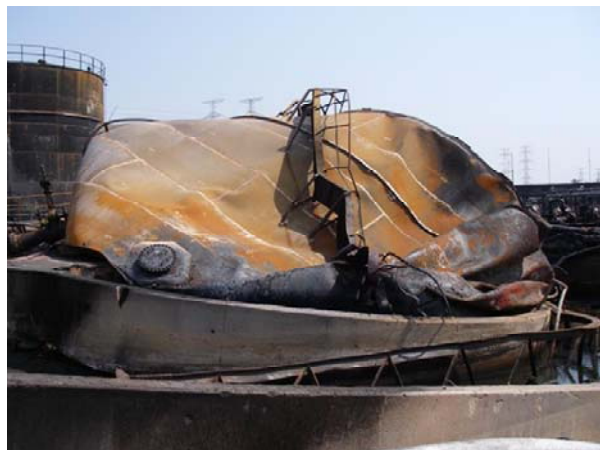
Figure 6. Burned-out gasoline tank
