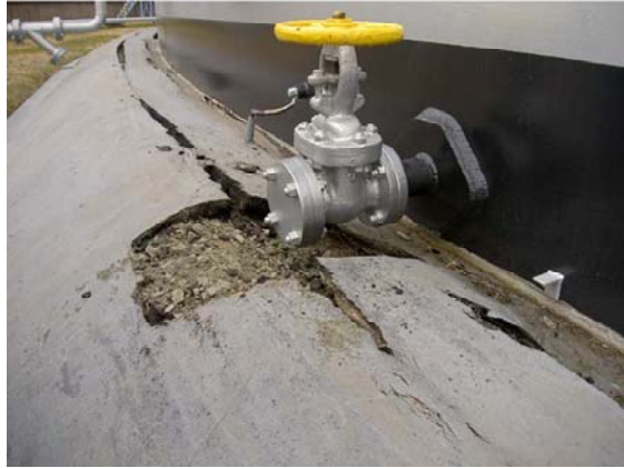
Figure 16. Tank settlement due to the liquefaction around the foundation
